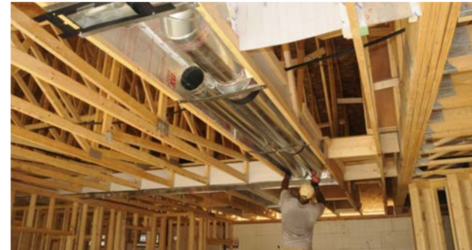
Figure 40 : Ductwork. (Source : Crowl Marketing + creative courtesy Pro Builder Media https://www.probuilder.com/ )
